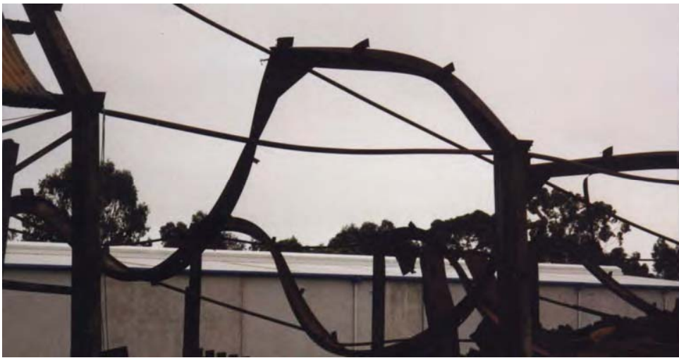
Figure 2.7 Remains of a steel framed building gutted by fire, Ashmore, Gold Coast
