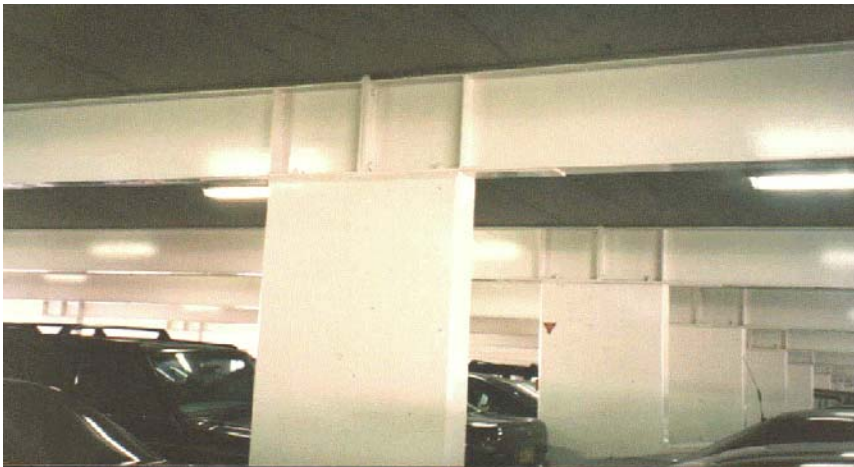
Figure1.5 Composite construction: steel beams supporting concrete slab in Sydney Airport car park
